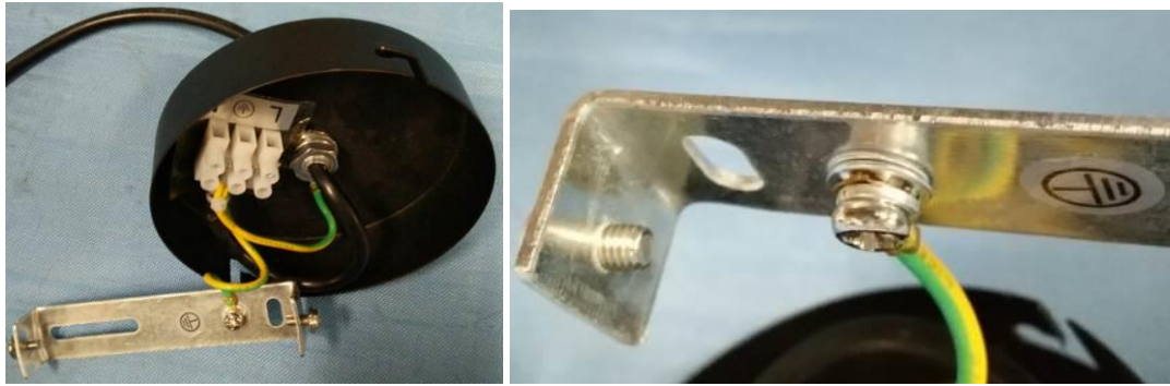
Photo 31: earthing connection view for model LS-PE863
