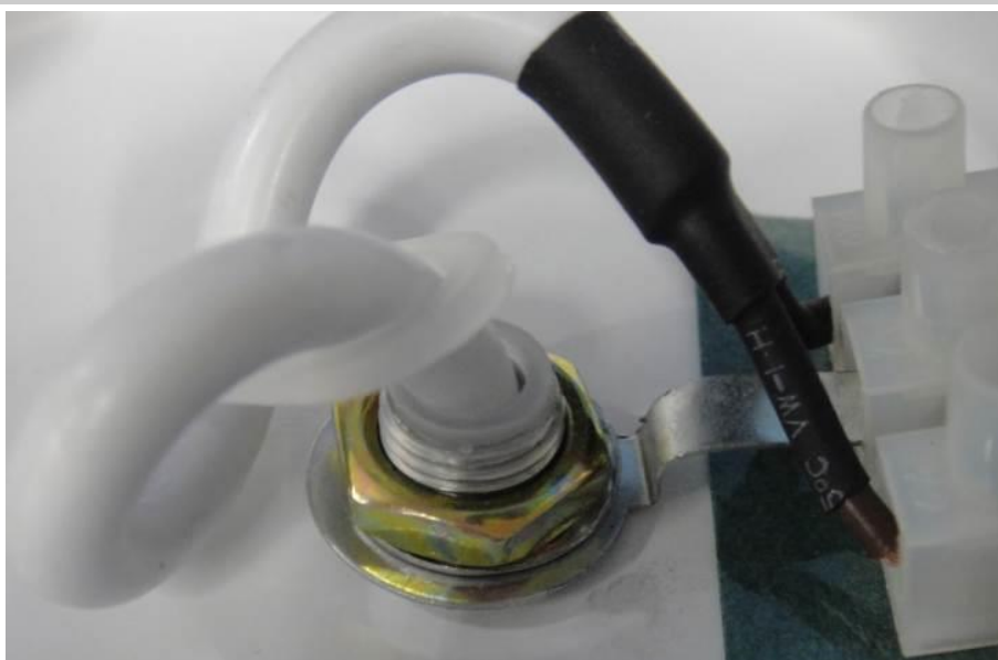
Photo 53: earthing connection view for model LS-PE0010
